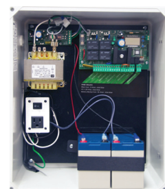
12 x 14 LEB enclosure with battery backup
