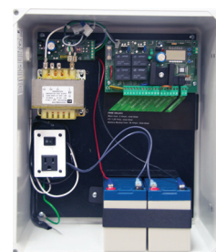
12 x 14 LEB enclosure with battery backup
